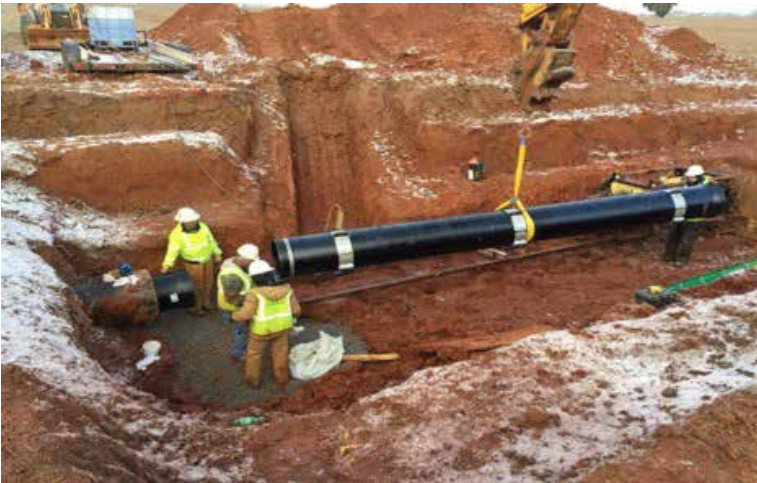
Fort Campbell, Kentucky: Resilience through redundant water supply and elimination of water leaks (UESC)
