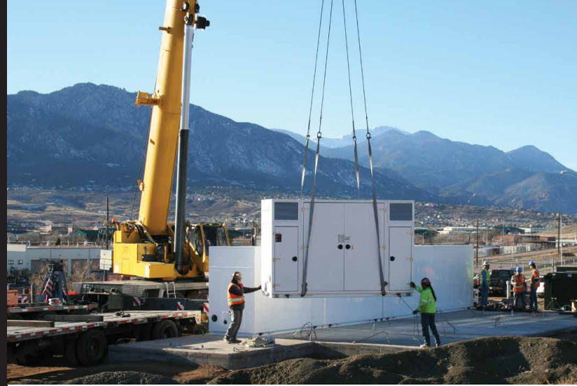
Ft. Carson Battery Energy Storage System (ESPC)
