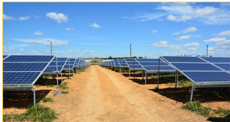
15 MW Solar Facility Comprised of 59,994 Solar Panels at Fort Detrick, MD
