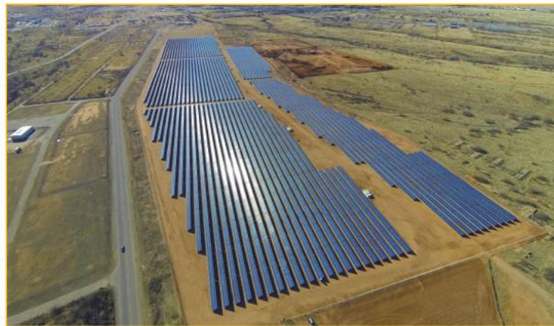
Fort Huachuca, AZ, 18 MW solar array; 103,900 solar panels
