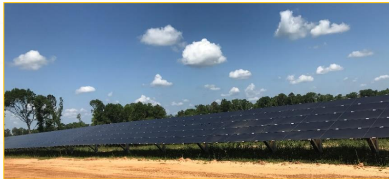
The 10 MW solar array at Fort Rucker, AL, is comprised of more than 115,000 solar panels.
