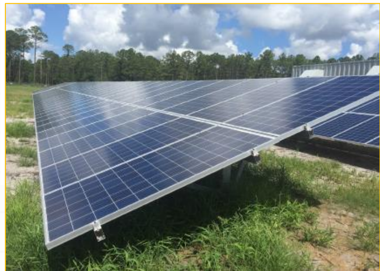
Fort Stewart, Georgia, 30 MW solar array, 137,640 solar panels
