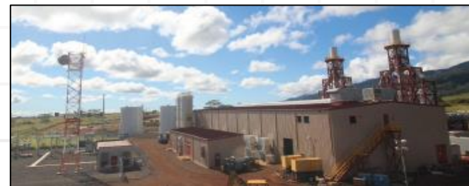
Schofield Barracks, HI: Lease Project: 50 MW / 30 day contingency microgrid where Hawaiian Electric constructed, owns, operates and maintains a 50 MW multi-fuel power generation plant, fuel storage tanks, and controls.
