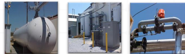
Anniston Army Depot, AL: UESC Replacement and Modernization of Depot-wide central heating and process high pressure steam plants, HVAC equipment and controls, interior and exterior lighting, compressed air equipment and distributions, and potable water fixtures.
