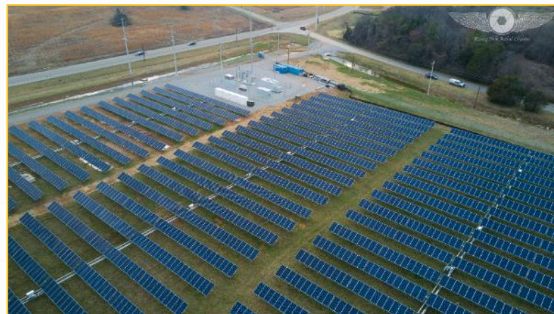
A 1 MW / 2 MW-hour battery energy storage system is coupled with a 10 MW onsite solar array at Redstone Arsenal, AL.
